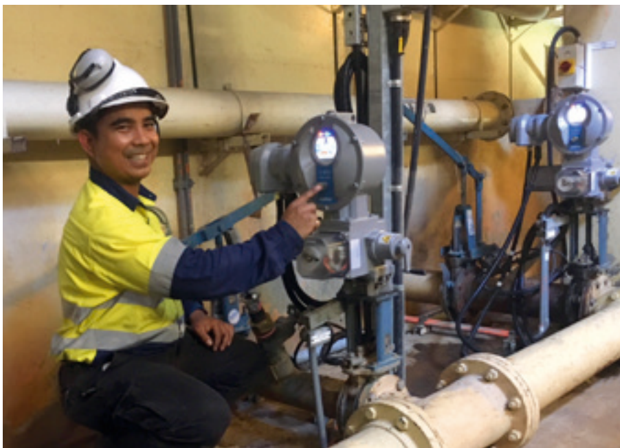
Sid Boholano of Barron GJM Ltd., AUMA's subsidiary in Australia, works on one of the 46 SEVEN actuators at Hornsby Heights Wastewater Treatment Plant
