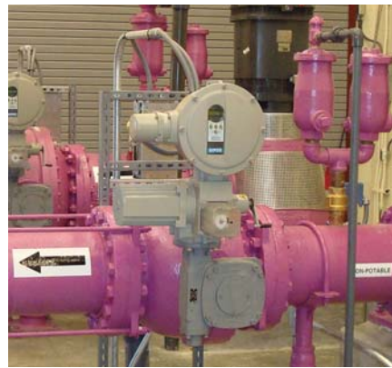
Figure 5: The topic of pressure surge reduction is a key consideration for pump station projects for Pipestone Equipment.
