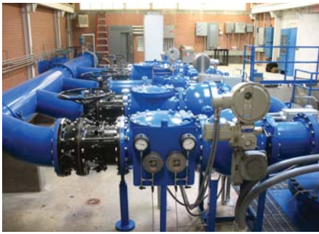
Figure 4: Pump station project - SIPOS 5 actuators controlling 16" ball valves are shown. Due to linear throughput control, the actuators ensure smooth pump operation.
