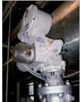
Bild 7: SIPOS-Drehantrieb regelt den Dampfdruck bei Baekert Steel Wire, Steam Installation/BE Fig. 7: SIPOS rotary actuator controlling steam pressure at Baekert Steel Wire, steam installation, Belgium
