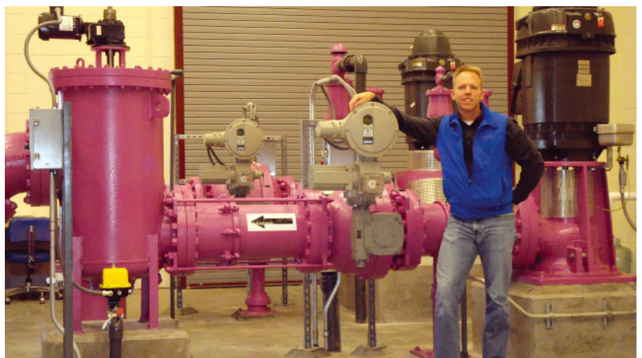
The North Water Reclamation project at Erie is the latest in a series of installations that confirms Pipestone Equipment's expertise in project management
