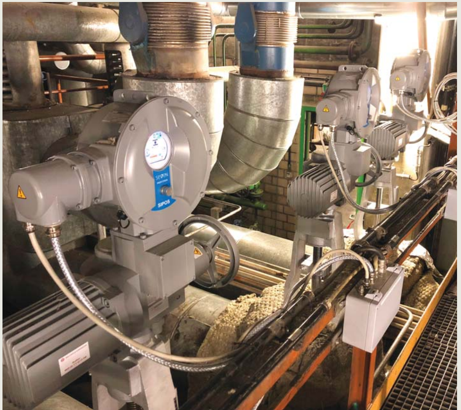
SIPOS SEVEN actuators ensure precise control of steam pressure reduction valves by Welland & Tuxhorn at the Sandreuth CHP plant.
