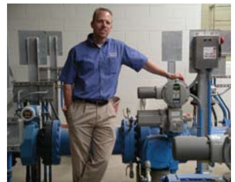
Water hammer is controlled at East Cherry Creek
