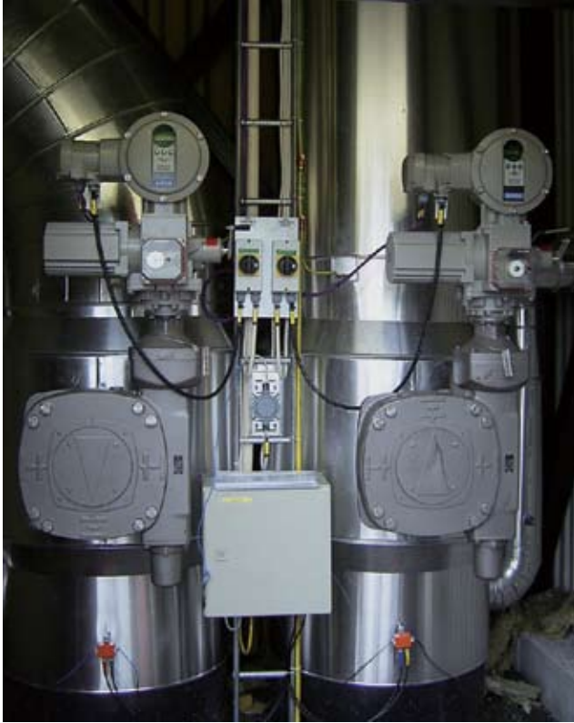
一个区域供热泵站的SIPOS 5 阀门 SIPOS 5 Flash in a district heating pumping station
